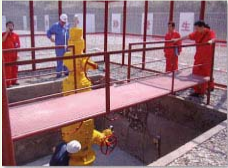
Many locations in the Chuandongbei gas development area have platforms built like this one for safe access to wellhead valves.
